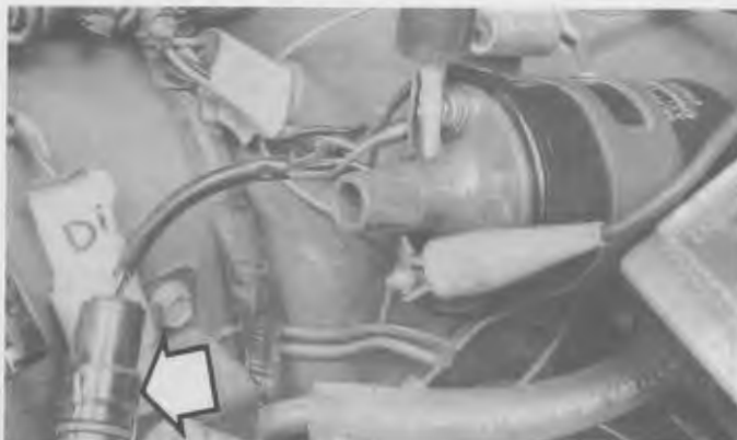
7.3a With the primary wiring electrical connector (arrow) unplugged, check the resistance across the primary terminals (1990 and earlier models)
